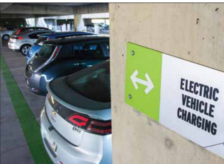
NREL employees charge their PEVs at the company's parking garage.
